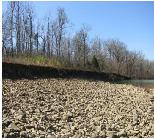
Eroding streambank on the Fourche La Fave River.
